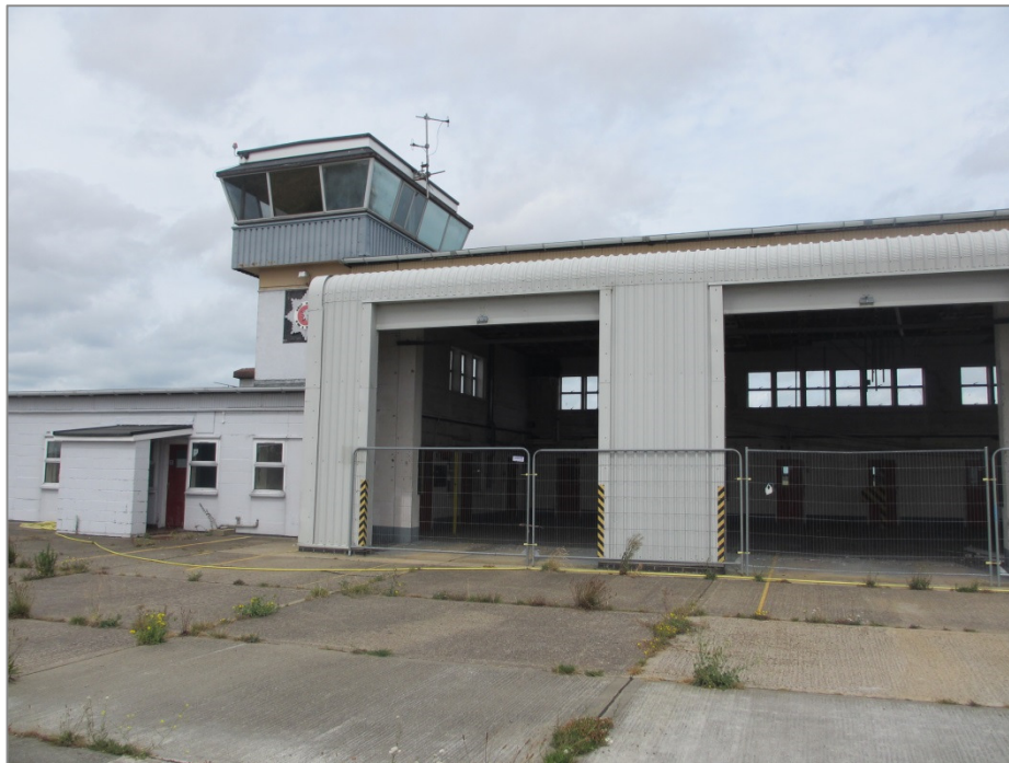
Figure 13: Dilapidated Rescue & Fire Fighting Facility
